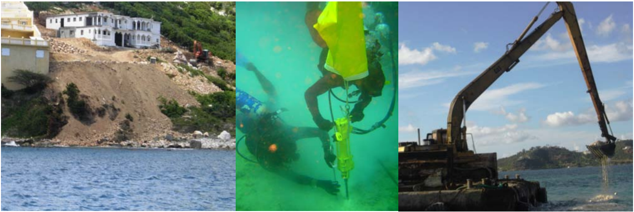
Group image 2. Poor terrestrial excavation practices as an earth mover shoves piles of soil over the cliff into the sea below; staff drilling seafloor to install mooring pin as part of the mooring maintenance programme; excavation in the marine environment without a permit and lack of sedimentation control measures.
